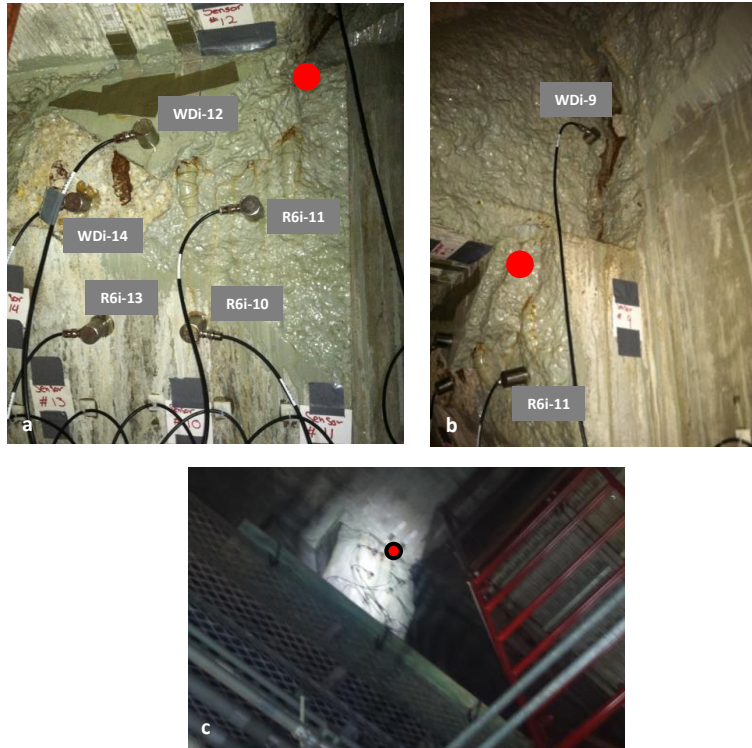
Figure 5.2 Photographs of the crane maintenance area: (a) main sensor grid, (b) close-up of sensor on side of column, and (c) view of main grid from floor level (red dot is at corner).
